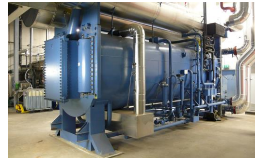
Industrial heat pumps and electrode boilers
